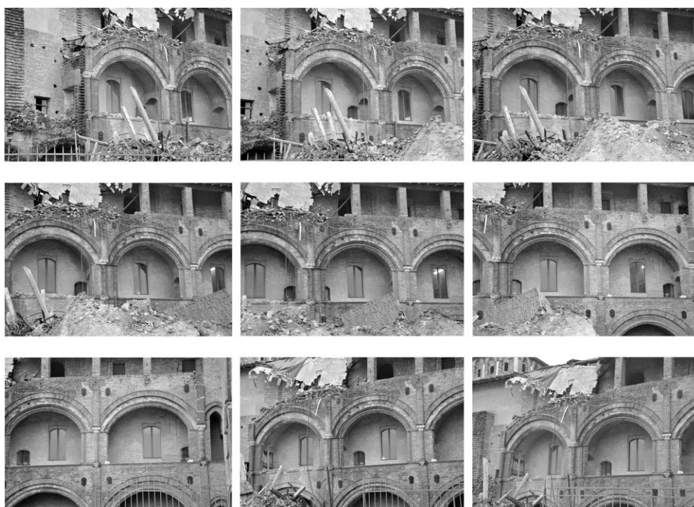
Fig. 1. Frames relative to the loggia of Finale Emilia Castle Fortresses damaged by the earthquake that hit
